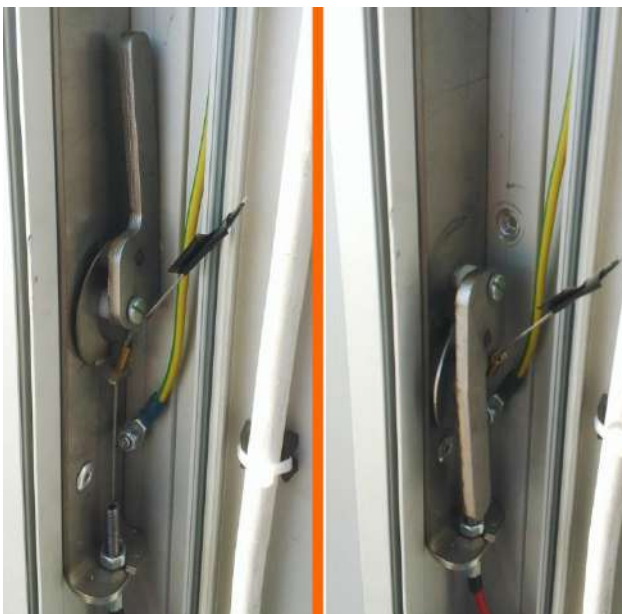
Not tripped – the handle is up. Platform control is functioning Tripped – the handles down. Platform control is not possible
